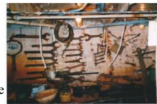
Engine room LV76 Spring 2005
